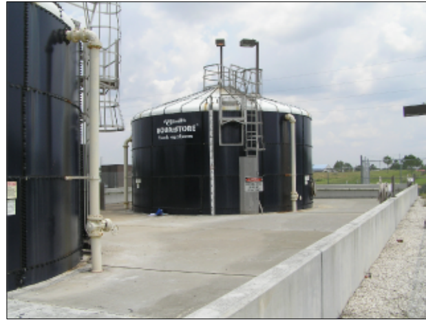
PARTIAL WEST TANK AND EAST TANK VIEW C M-1
