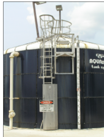
WEST TANK LADDER AND LEVEL INDICATOR VIEW
