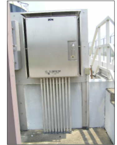
LEVEL TRANSMITTER ENCLOSURE VIEW D E-1
