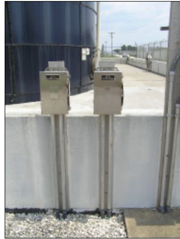
DISCONNECT SWITCHES VIEW A E-1
