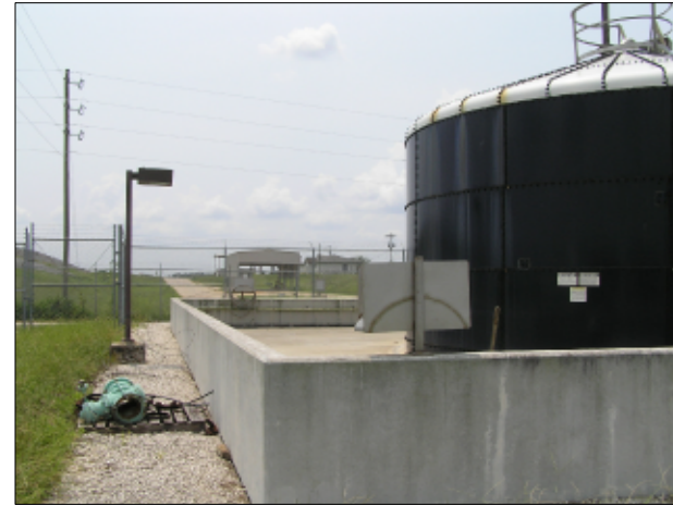
SIDE OF EAST TANK ALONG EAST CONTAINMENT WALL SOUTHWARD VIEW C E-1
