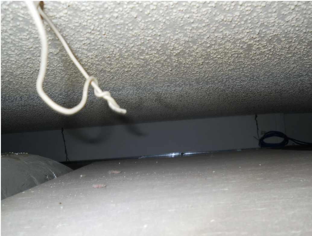
PHOTO 13 – 9/29/21 – APPARENT AIR EROSION AND DELAMINATION CEILING TREATMENT ABOVE ROOMS 24 AND 25
