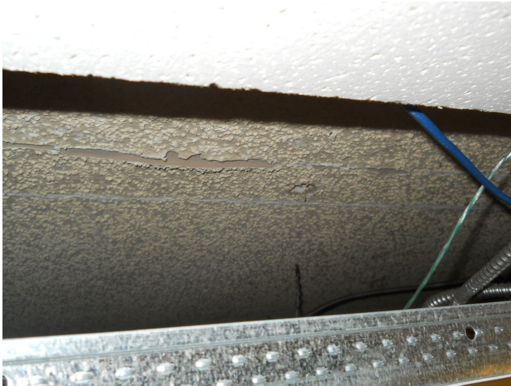
PHOTO 11 - 9/29/21 – PEELING CEILING TREATMENT SOUTHERN PORTION OF THE BUILDING
