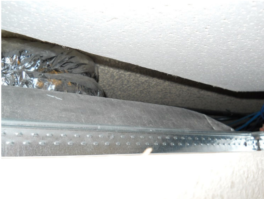
PHOTO 7 – 9/29/21 – APPARENT AIR EROSION OF CEILING TREATMENT IN THE EASTERN HALLWAY
