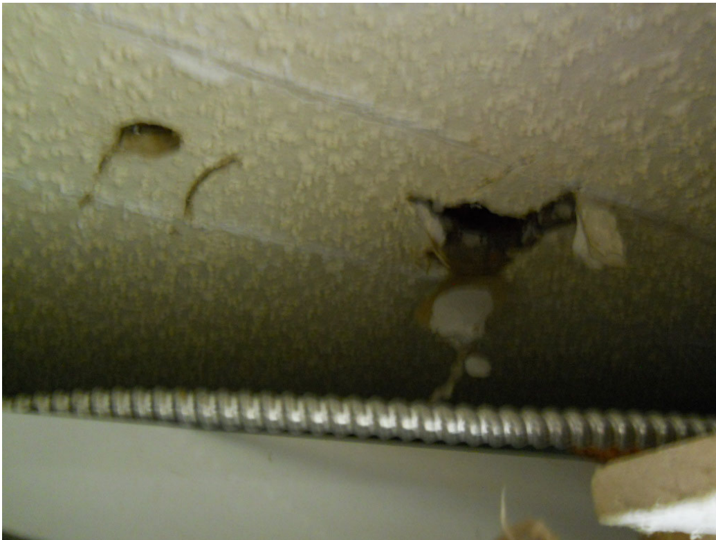
PHOTO 10 – 9/29/21 – LOCALIZED DAMAGE AND AIR EROSION OF CEILING TREATMENT ABOVE CUBICLE 31
