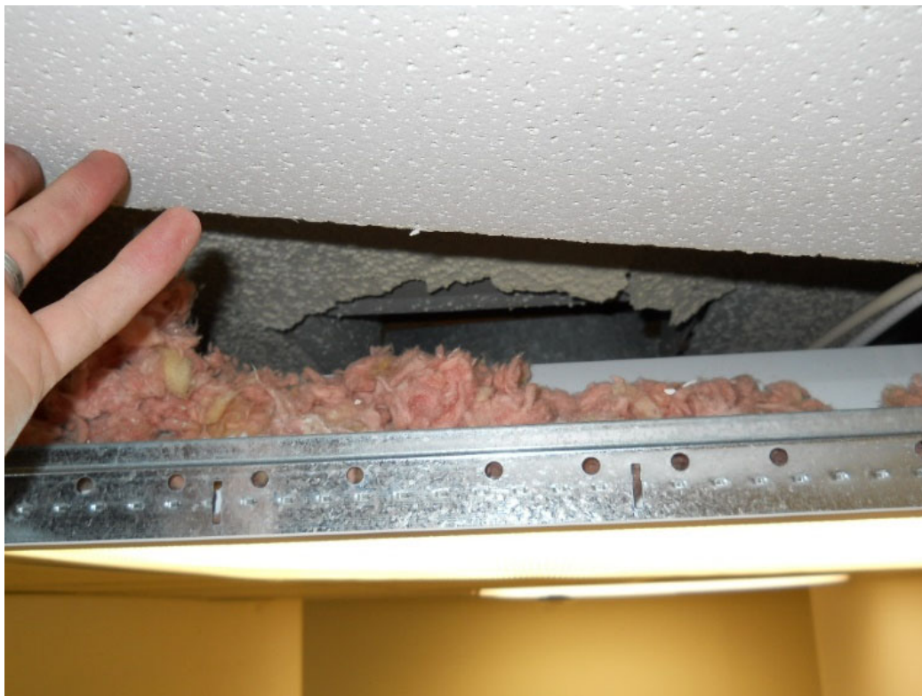
PHOTO 8 – 9/29/21 – LOCALIZED PEELING CEILING TREATMENT IN THE EASTERN HALLWAY
