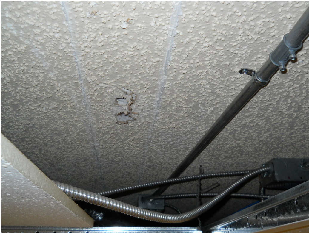
PHOTO 9 – 9/29/21 – LOCALIZED DAMAGE AND AIR EROSION OF CEILING TREATMENT ABOVE ROOM 15
