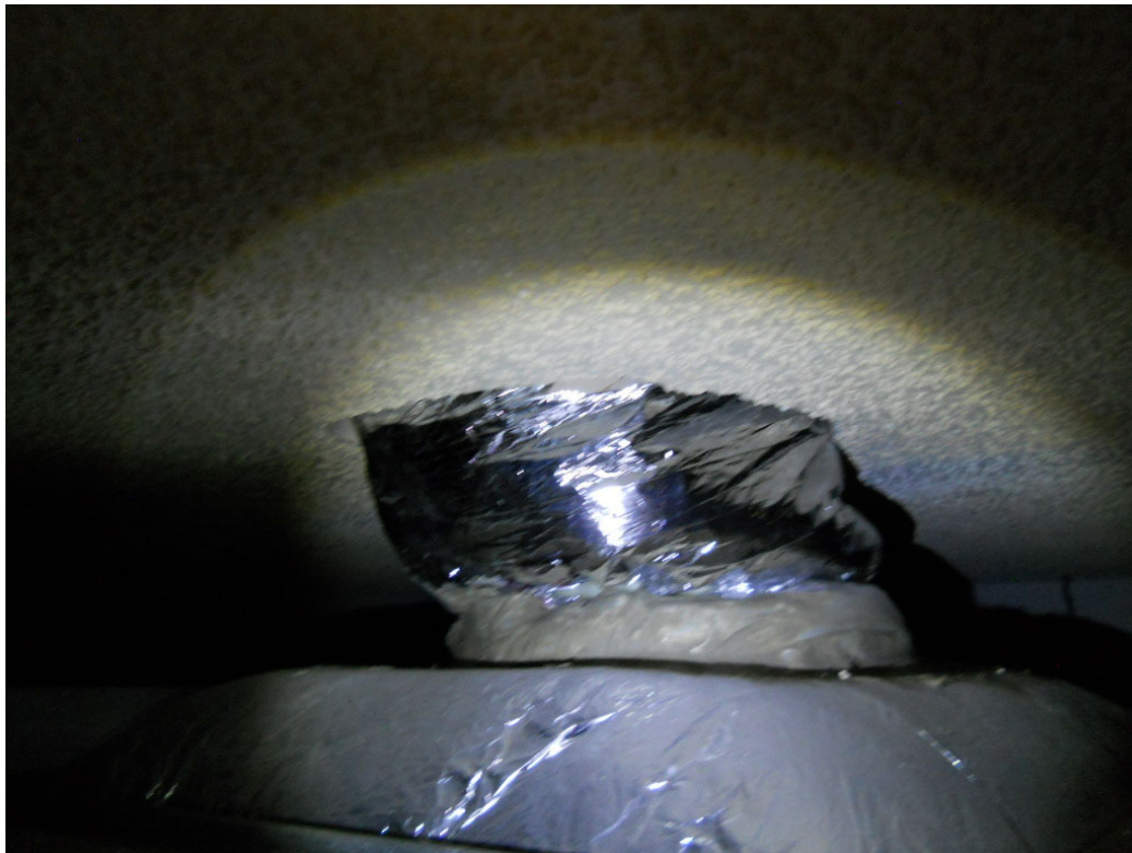
PHOTO 12 – 9/29/21 – PEELING CEILING TREATMENT CEILING TREATMENT ABOVE ROOM 23
