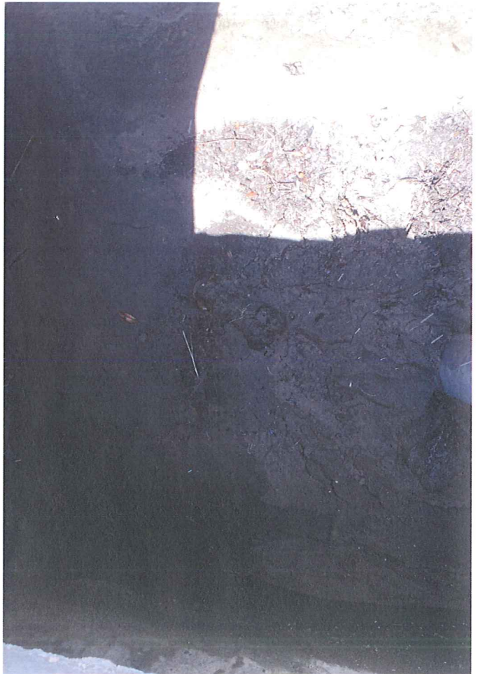
Cement Inlet south
