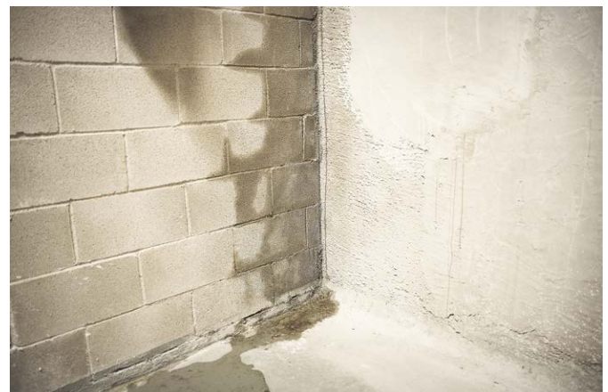
Subsystem level water intrusion
