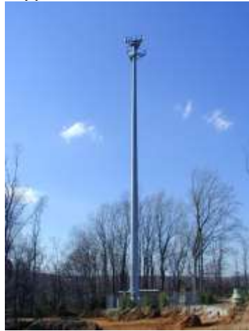
Typical Mono-Pole Tower
