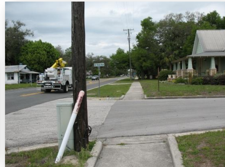
The intersection of SR 471 and S.E. 3 rd Avenue lacks stop bars and crosswalks
